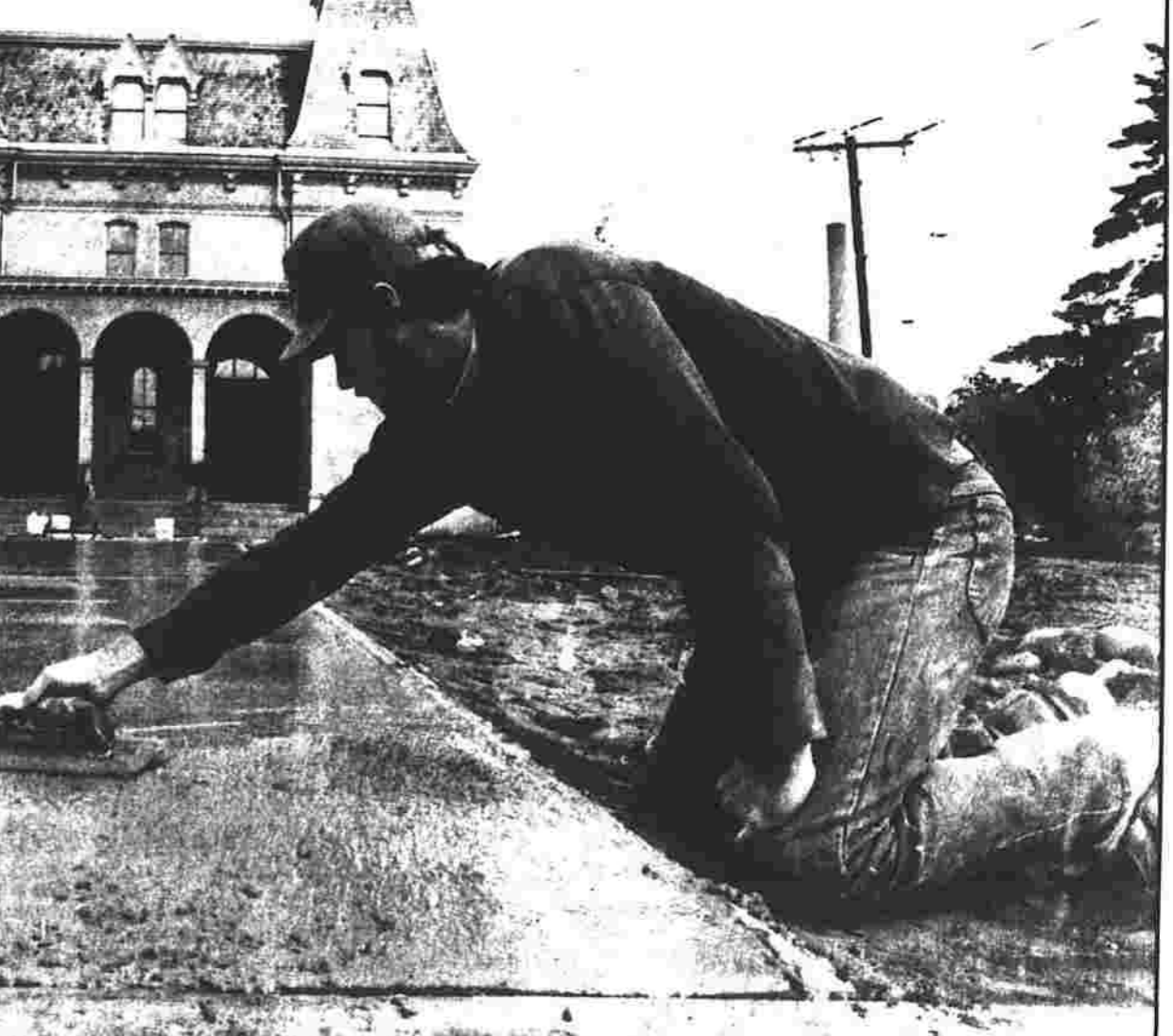
Fred Spoor of Lebanon, Conn., smooths the cement on a new sidewalk in front of Manchester's Cheney Hall. The historic structure on Hartford Road is in the middle of a restoration and renovation project. The sidewalk work was being done this morning by Milton Beebe and Sons Inc.
